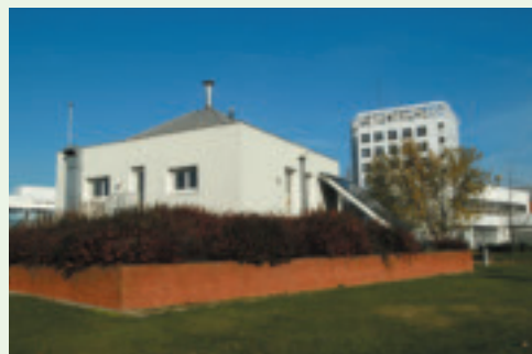
Electrical room with connections for the combined heat and power plant installed at OPAC, Paris, France. Gaz de France.
