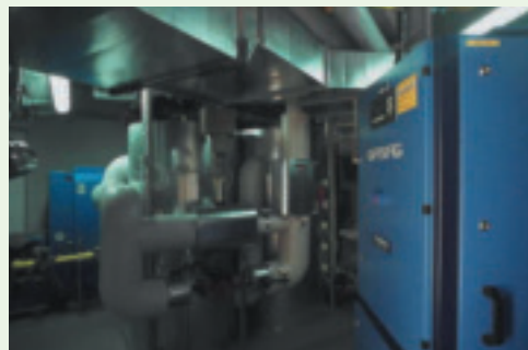
A cogeneration boiler at Emmentalerstrasse, Berlin, Germany. Gaz de France.
